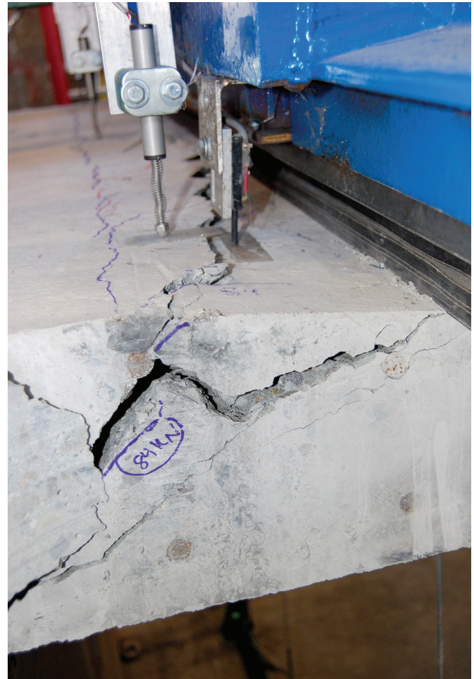
(b) Diagonal crack on edge going below concrete cover
